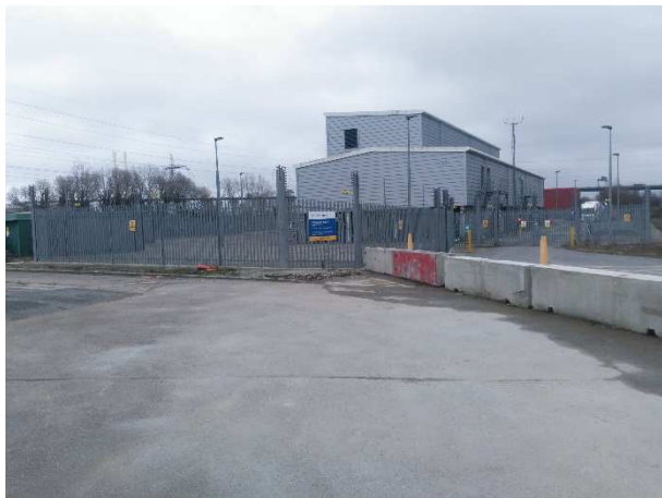
Plate 30 – Littlebrook 132kV substation
